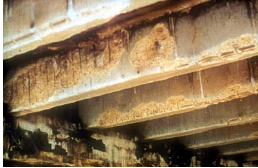
Figure CS1.2 Example of concrete elements after the fire showing spalling. (Courtesy DBV, Germany)
